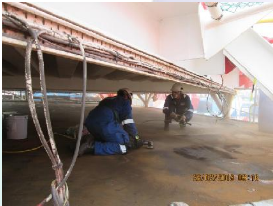
Pic 3: Air Powered Twist knot wire brushes were used to remove the build-up of oxidisation that had occurred.
