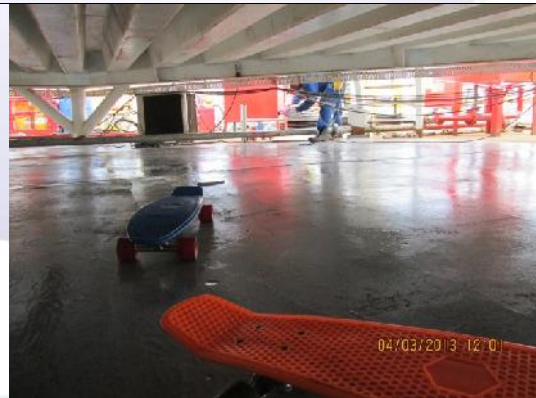
Pic 10: Primed surface with transport system on view. Provided mobility in tight area.
