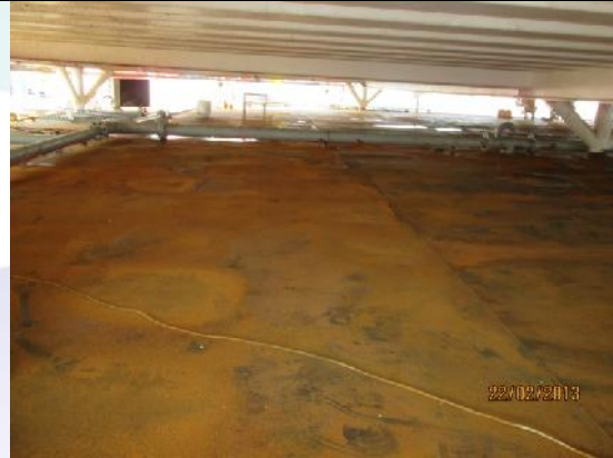
Pic 2: As per previous pic, surface oxidization had reached critical levels over two week period must be removed.
