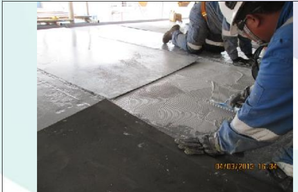
Pic 14: Plate ready for laying down onto bed whilst it is wet,
