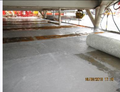
Pic 19: Laminating completed in every second strip to give access whilst the application is on-going.
