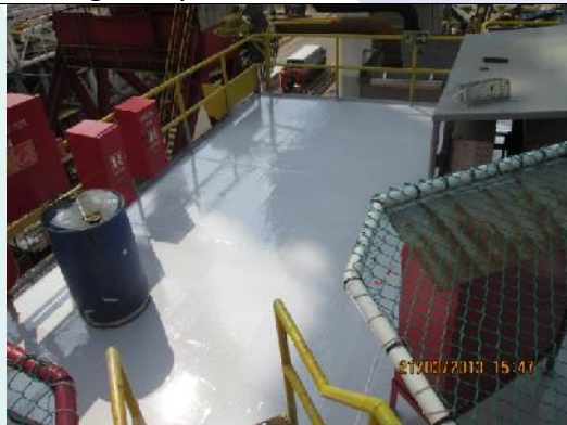
Pic 27: Several other external areas were completed to finish off entire deck
