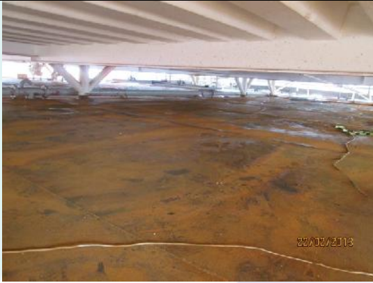
Pic 1: Surface Before the treatment after the high pressure water blast as carried out by the shipyard.
