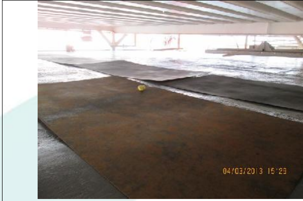
Pic 11: Plates bought on to site they have been blasted on the side facing the deck, for maximum adhesion
