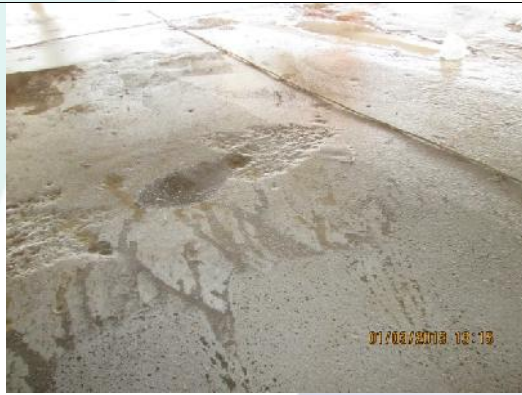
Pic 7: Surface pitting severe in several places.
