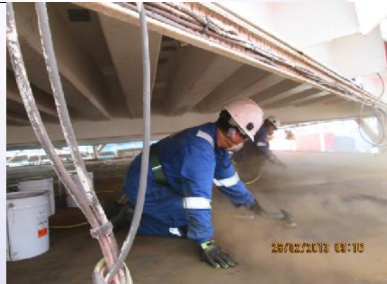
Pic 4: Heavy Oxidisation being removed by Power Wire Brush ready to prime after washing
