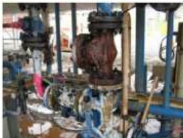
Before – Ammonia Bullet Pipelines
